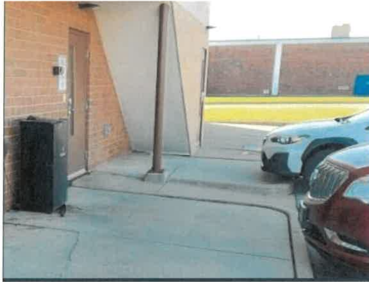
Non-Compliant Accessible Entrance Ramp
