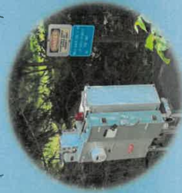
Mission Remote Terminal Unit (Brindlestone LS)
