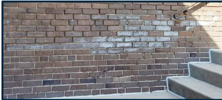
Efflorescence on Building Wall
