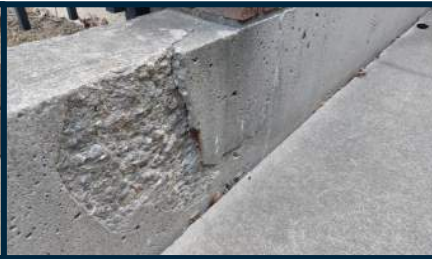
Spalling at Mech Enclosure
