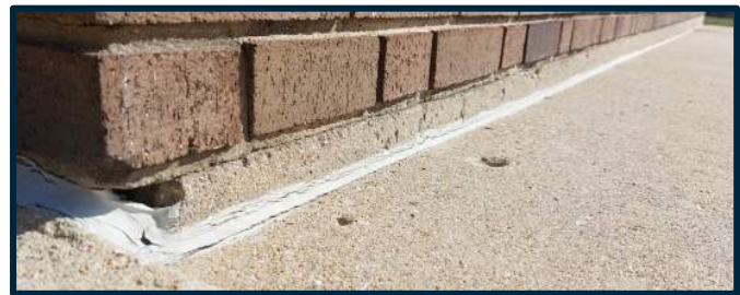
Aging Perimeter Sealant
