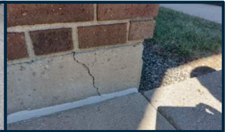
Foundation Cracks at Building Corners
