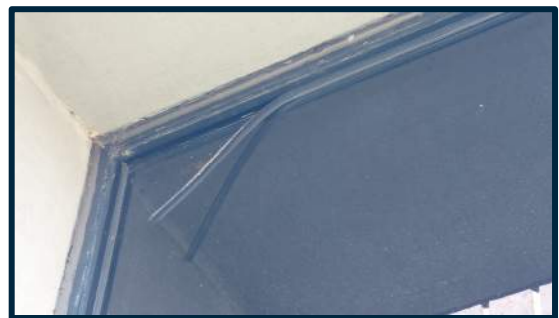
Loose Window Gasket
