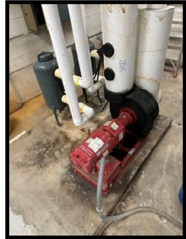
Chilled water pump
