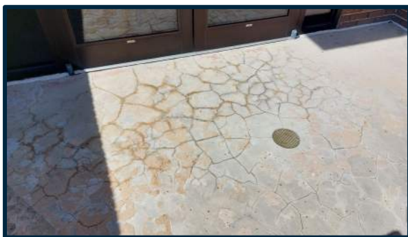
Cracked Leveling Compound
