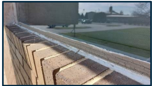
Weathered Window Glazing
