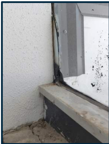
Broken Pane of Glass
