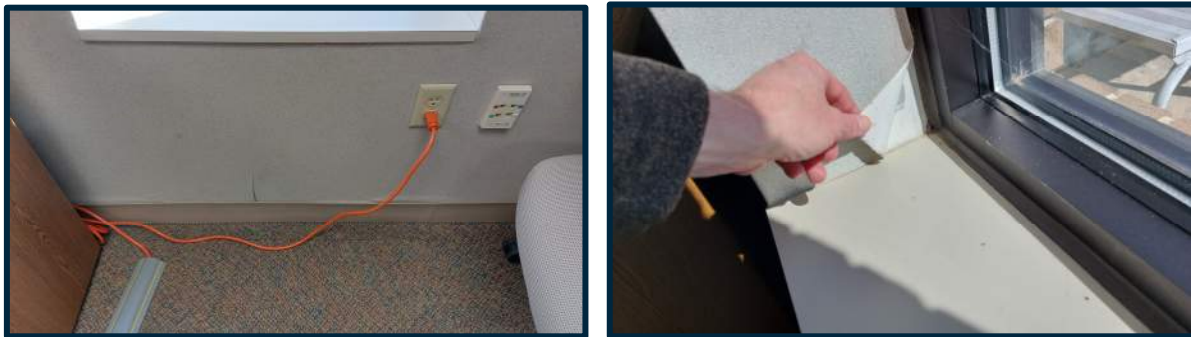
Engineering Conference Room Window
