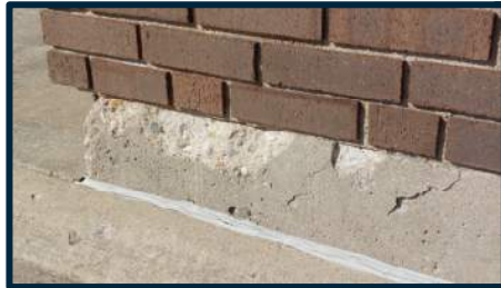
Chipped Conc around Top of Foundation
