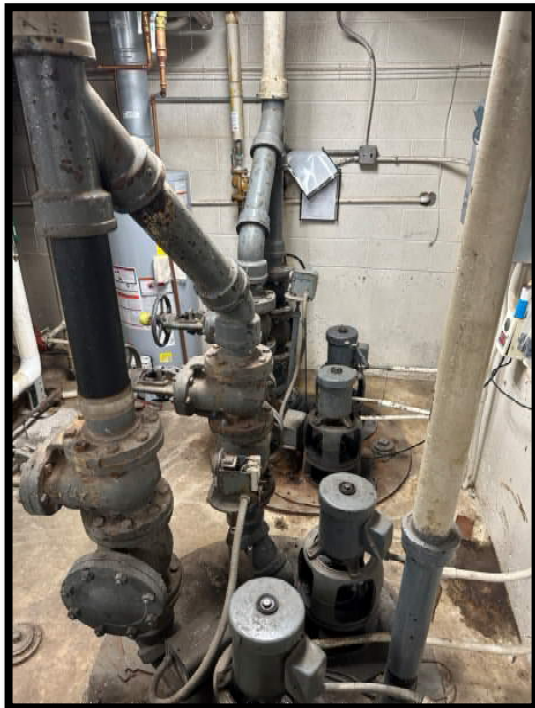
Sewage Ejector and Sump Pump Stations
