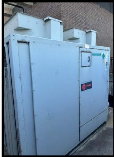
Existing Air Cooled Chiller prior to removal
