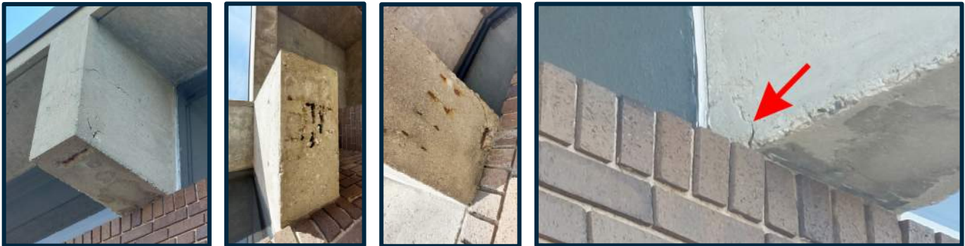
Cast-in-Place Joist System Deterioration
