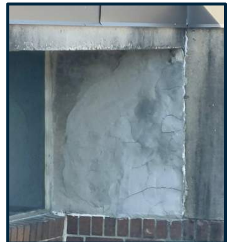
Failing Patch within the Cove of the Antenna Tower
